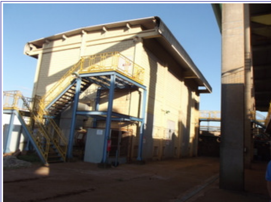
CCM GRINDING SUBSTATION
