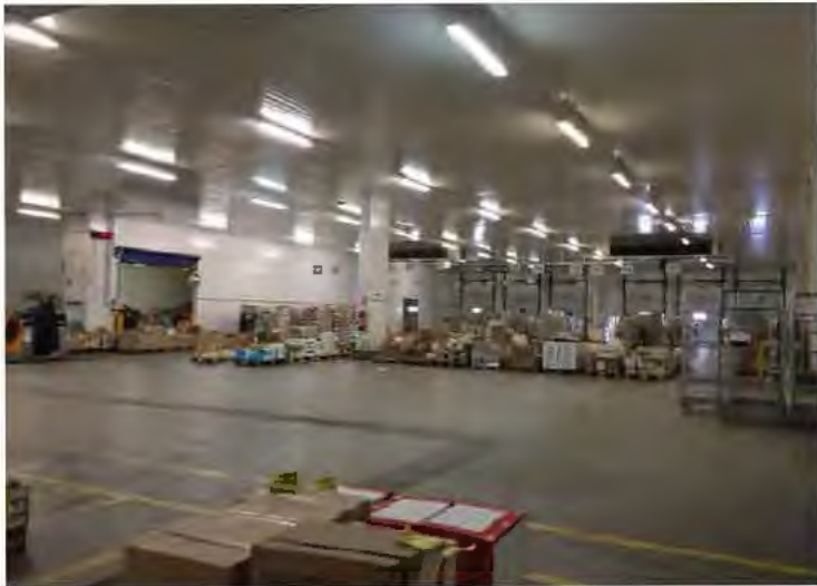
Warehouse positive cooled areas
